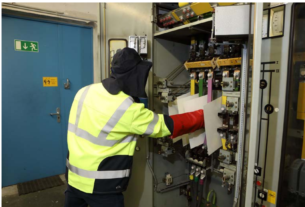
Fig. A 5-20 Removal of NH fuse-links, additional portable separators to isolate different potentials
