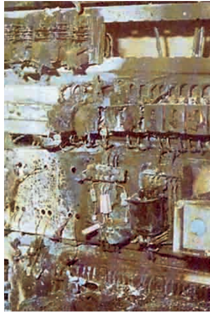
Fig. 3.1: Installation after an electric arc accident (source: Schau)
