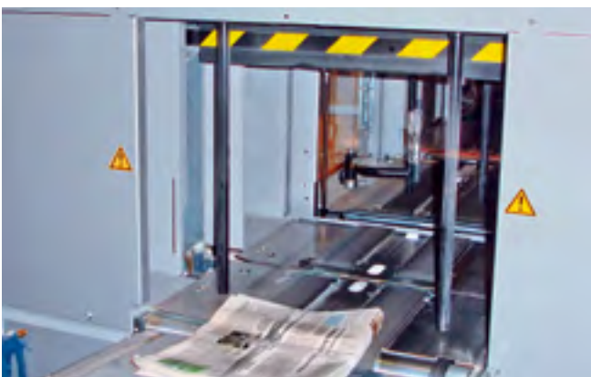
Safeguarding the crushing point between hold-down and news-paper package by limiting the force and providing foam rubber padding on the upper and lower side of the clamping bar for finger protection
