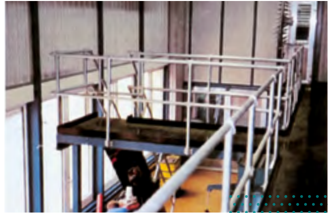
Fall-off protection on machine access by locating stairs sideways
