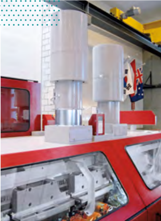
Exhaust equipment with activated carbon filter on a perfect binder
