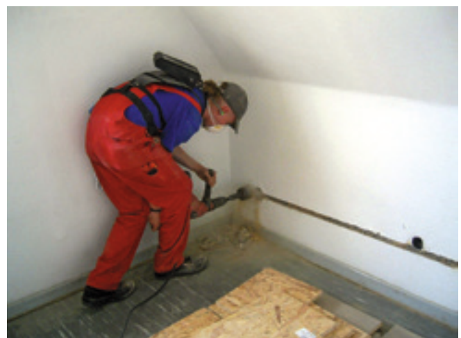
Drilling flush sockets without suction with a clearly recognisable source of dust formation
